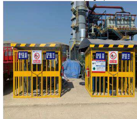
Gas cylinder storage
