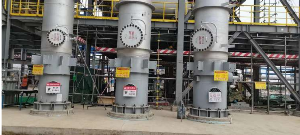
Safety warning signs of confined space
